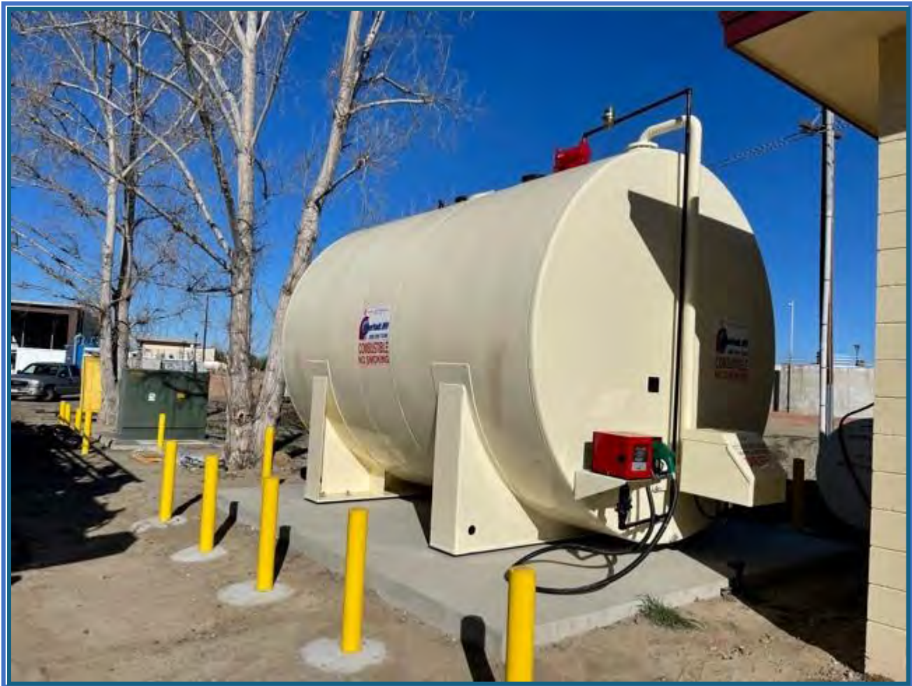
Emergency Fuel Tank
